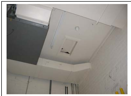
Left: manhole cover – damaged asbestos sheeting
